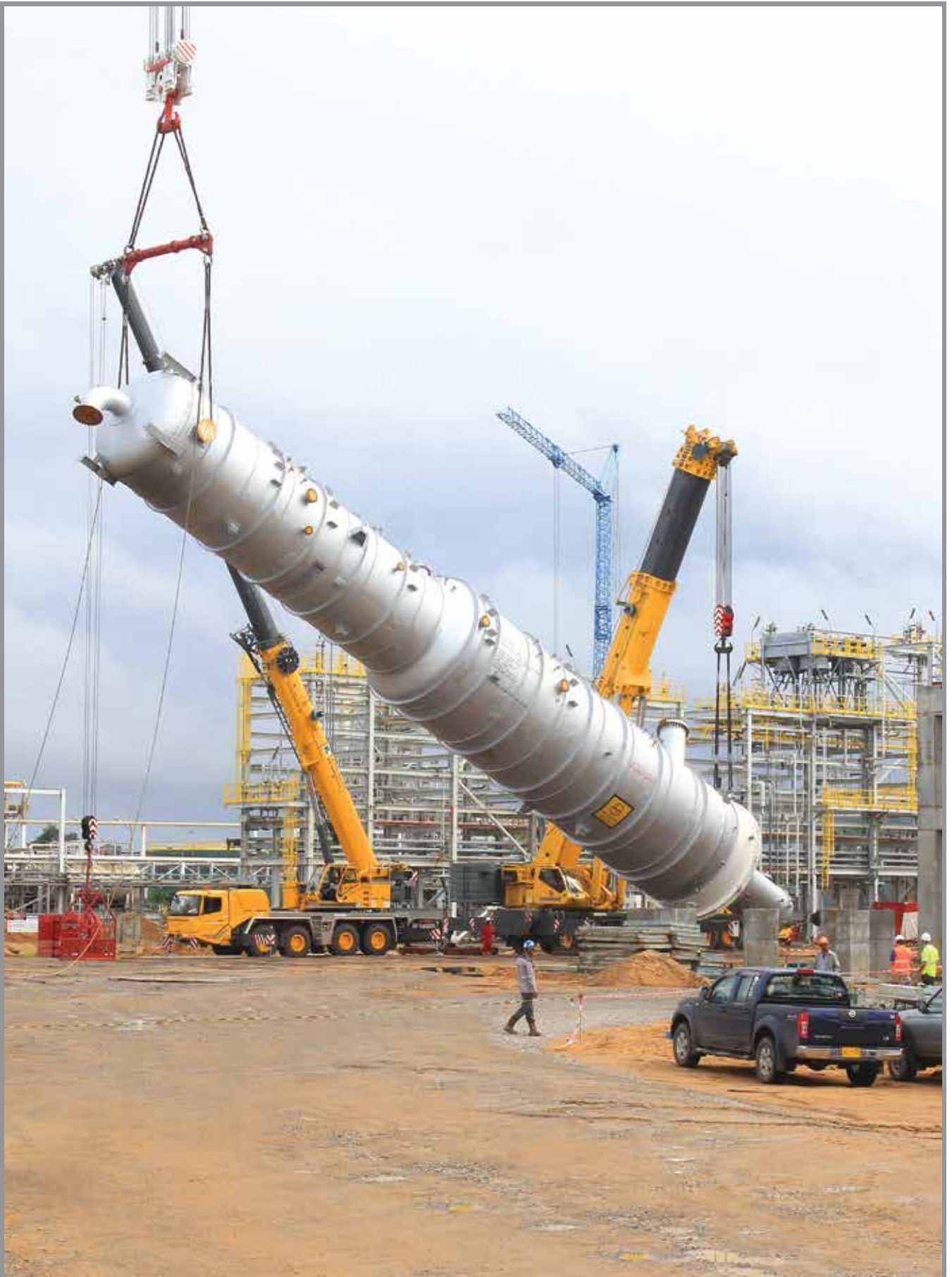
Work in progress at the Refinery Expansion Project. The vacuum tower is placed on its foundation.
